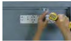
Replacement Plate installed reusing the existing holes in the door. No need to drill new holes.
