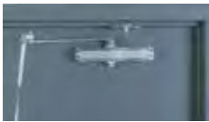
Old door closer needing to be replaced.
